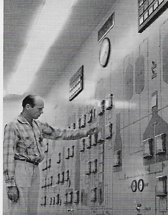
Finally Operator Rue adjusts an instrument in the control room, putting the dual unit on stream.
