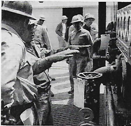
A long-earned week is at hand—start-up! Under engineering direction, a blower adds its low hum to the gentle refinery chorus;
