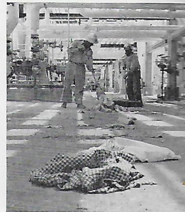
construction debris is swept out, providing a working area that is neat and devoid of any accident hazards;
